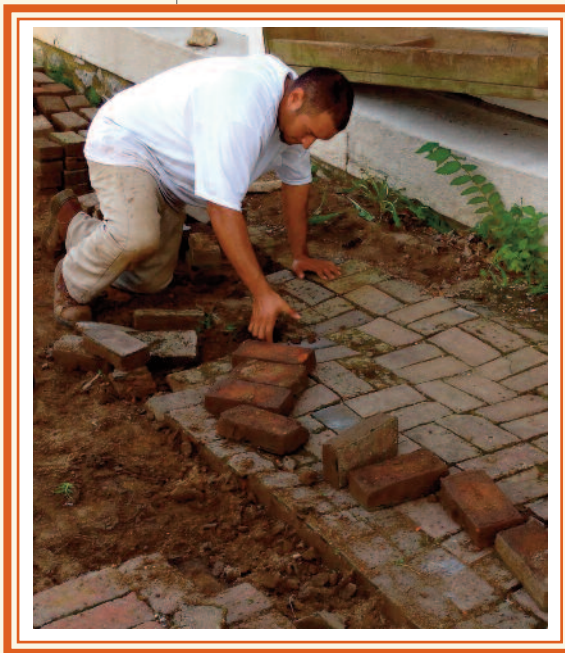
Rico Palacio of Pishny Restoration Services removes the uneven brick sidewalk in front of the Odd Fellows Lodge to prepare for a safer, level walk.
