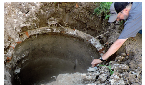
LEFT: Properties Manager Marty Selby inspects the progress of the cistern removal behind the Sites Gunsmith Shop.
