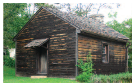
A new roof will go on the Log Cabin thanks to a grant from the A. P. Green Foundation.
